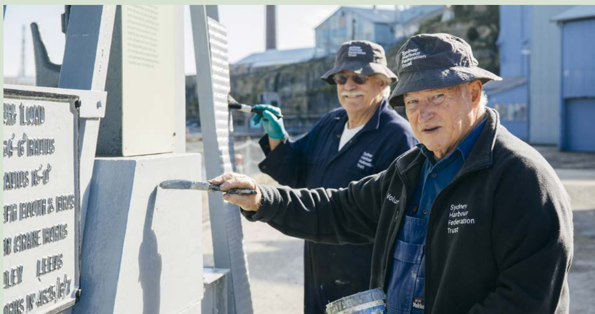
Cockatoo Island heritage restoration volunteers painting the Mort's Dock Steam Crane, Fitzroy Dock, Cockatoo Island, New South Wales Photo by Zakarij Kaczmarek, courtesy of the Sydney Harbour Federation Trust
