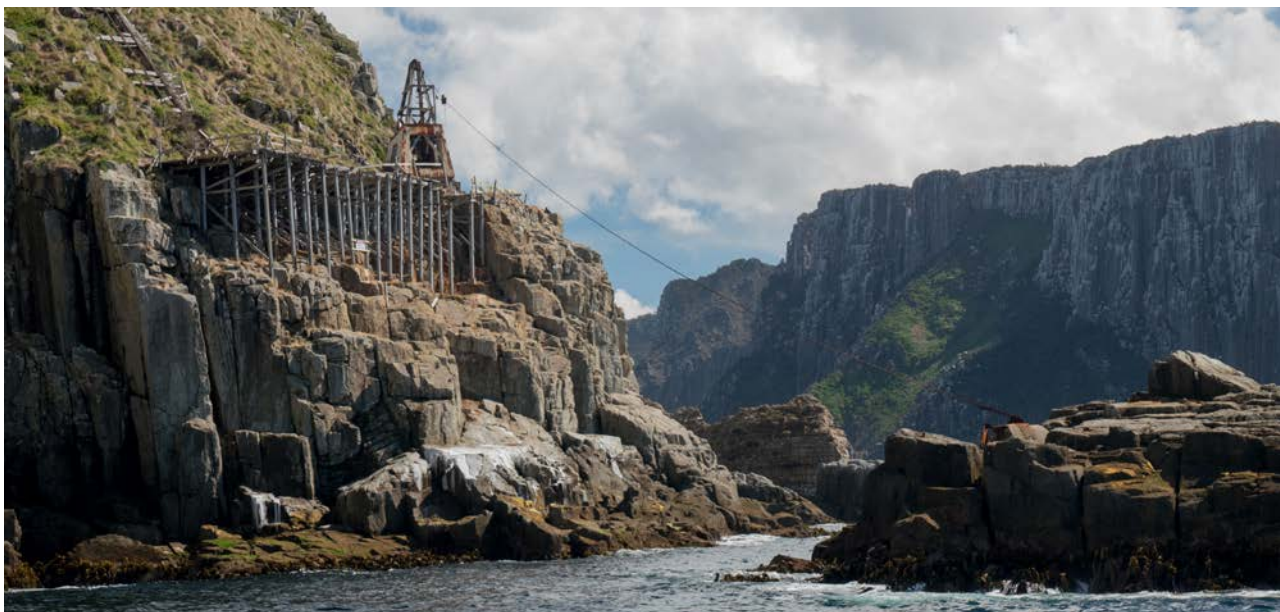
Tasman Island, showing winch used to move building materials for lighthouse construction
