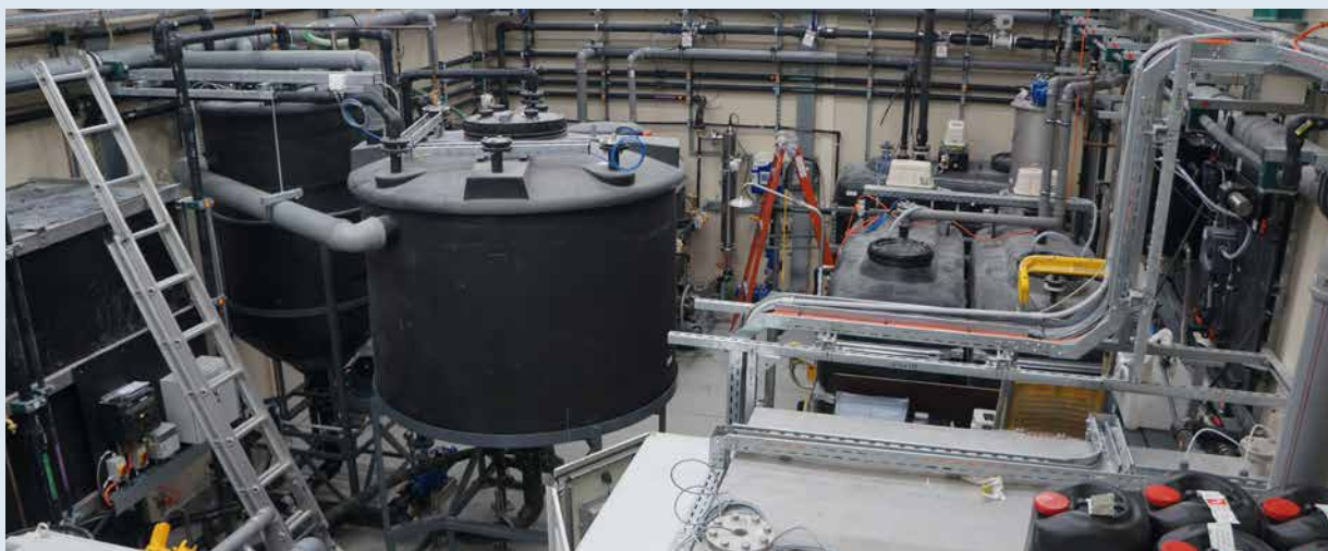
The secondary-level water treatment plant at Davis Station Photo by Michael Packer, Australian Antarctic Division, all rights reserved
