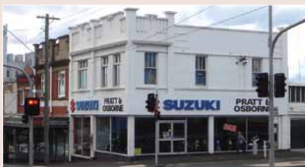
■ 231 Moorabool St, Geelong, before verandah reconstruction (photo by Michael Bell, Manifest Architects, Geelong)
