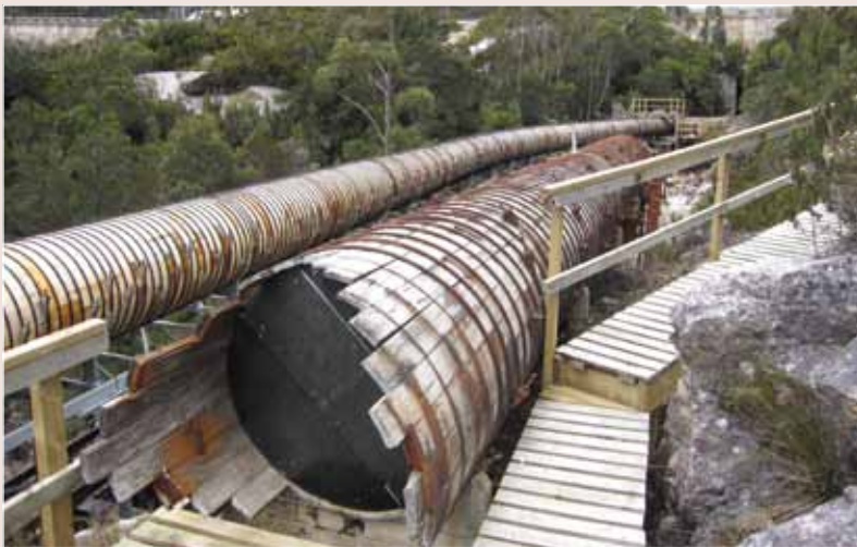
■ Section of the woodstave pipeline, Lake Margaret Power Station, Tasmania (photo by David Scott, Heritage Tasmania)
