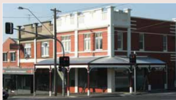
■ 231 Moorabool St, Geelong, after verandah reconstruction (photo by David Rowe, Authentic Heritage Services Pty Ltd, Heritage Adviser, City of Geelong)
